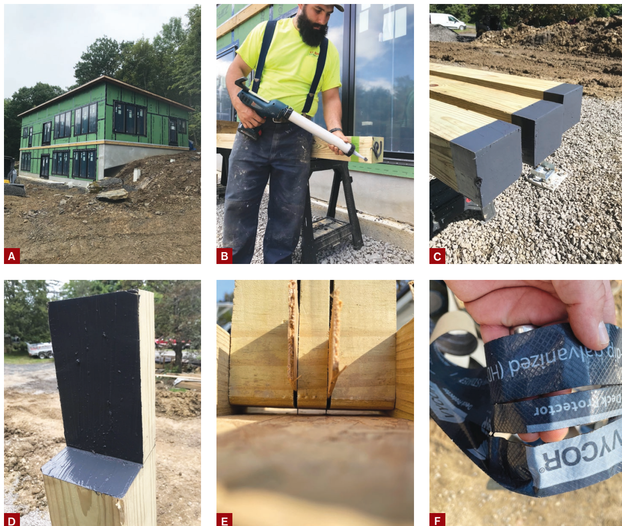
Figure 1. Precast concrete piers were installed to support the deck (A). Prior to installing the 6x6 support posts, Ed Backus applied liquid flashing membrane to the post bases (B, C) and the notches for a 2-ply dropped beam (D). Backus assembled a quick jig fitted with a couple of utility blades (E) to slice Vycor flashing tape to cover the tops of joists (F).
